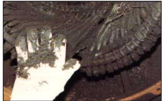
Motor Stator After Burnout
